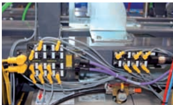
Turck Profibus AIM stations are used for I/O acquisition and control
