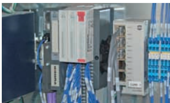
BL20 I/O systems installed within the subassembly give users control and diagnostics on the machine
